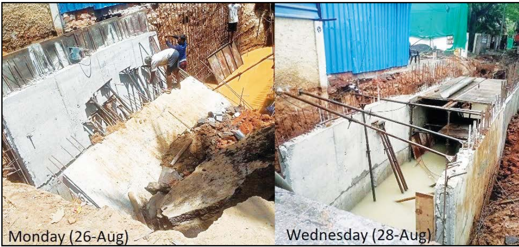
First photo shows collapsed drain wall. Second shows the scene after 'repairs'
